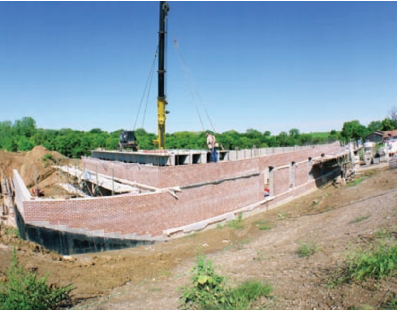
Project: Cernech Reservoir and Pump Station Location: Kansas City, Kan. Client: Kansas City Board of Public Utilities
