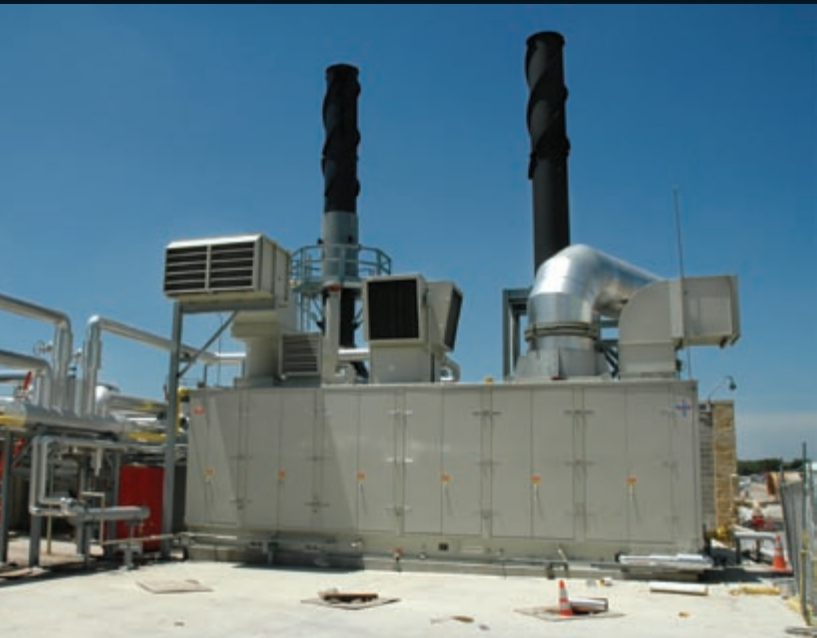
Project: Dell Children's Medical Center Location: Austin, Texas Client: Austin Energy
