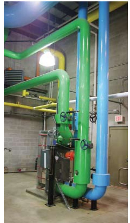
A new central heating and cooling plant for Wheaton College, Wheaton, Ill., incorporates a plate and frame heat exchanger (above) and two 600-ton centrifugal chillers (below left).
