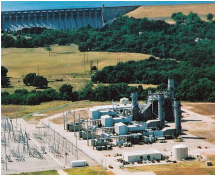
The conversion of Bosque Unit 3 from simple cycle to combined cycle was completed in just 14 months, shaving three to five months off a typical schedule and allowing Mirant to meet peak summer demand.
