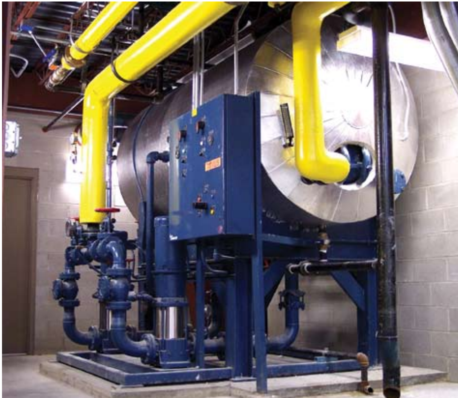
Wheaton College's central plant features chilled water pumps (top) and a surge tank and boiler feed water pumps.
