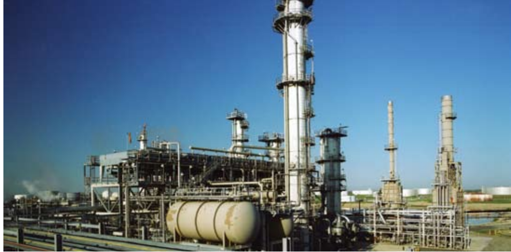
U.S. refiners are meeting requirements for sulfur and benzene, which were targets of the Environmental Protection Agency. Burns & McDonnell is currently helping seven refineries in the United States look for ways to meet benzene regulations.
