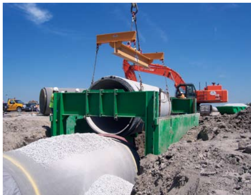
Project: Water Main Relocation Location: O'Hare International Airport, Chicago Client: City of Chicago
