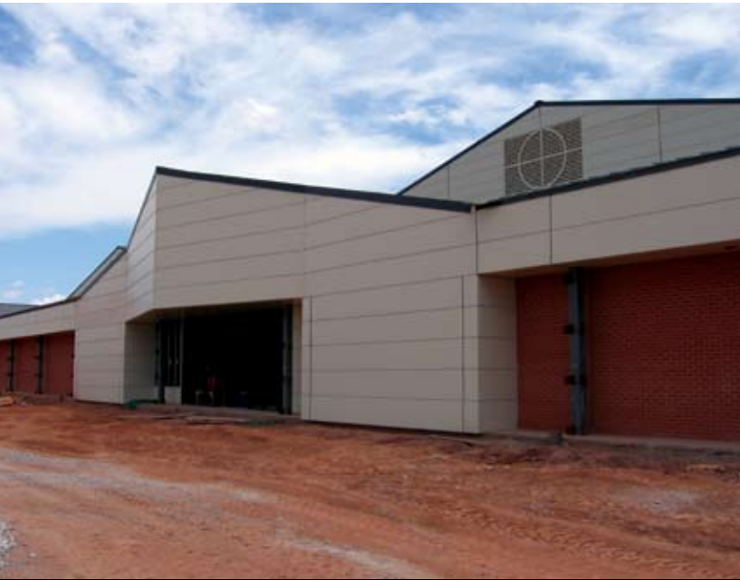
Project: F-22 Technical Training Facility Location: Sheppard Air Force Base, Wichita Falls, Texas Client: U.S. Air Force
