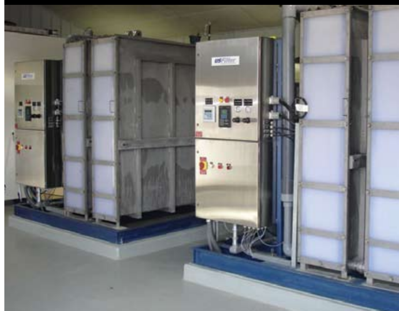
Project: Water Treatment Facility Location: Colorado City, Colo. Client: Colorado City Metropolitan District
