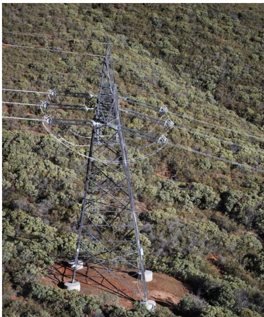
Figure 2: 500 kV transmission structure
