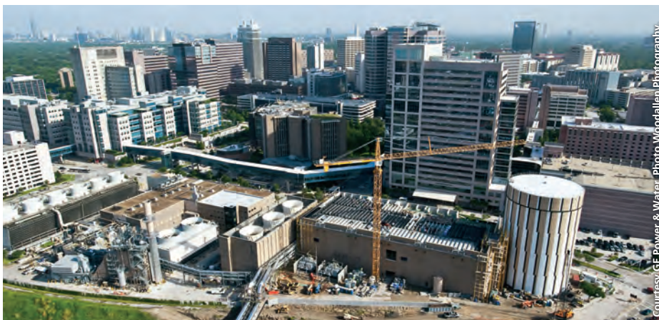
TECO's Central Plant site was under construction from 2008 until early May 2011. Nine months of construction remained when this aerial image with the Texas Medical Center campus in the background was captured. The expanded district energy facility's design allows TECO's capacity to reach 100 MW of on-site power generation, 168,000 tons of chilled water, 152,000 ton-hr of chilled-water storage and 940,000 lb/hr of steam.
