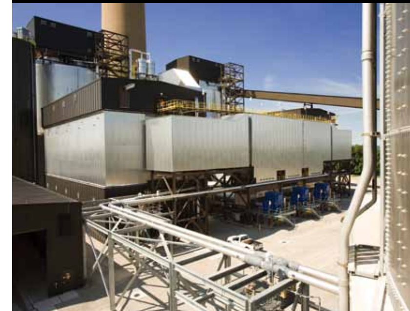
Project: Louisa Generating Station AQCS Retrofit Location: Muscataine, Iowa Client: MidAmerican Energy Co.
