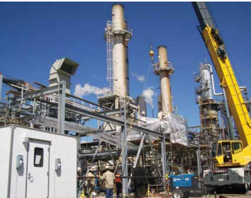
Project: Frontier Boiler No. 3 Location: Cheyenne, Wyo. Client: Frontier Refining Inc.
