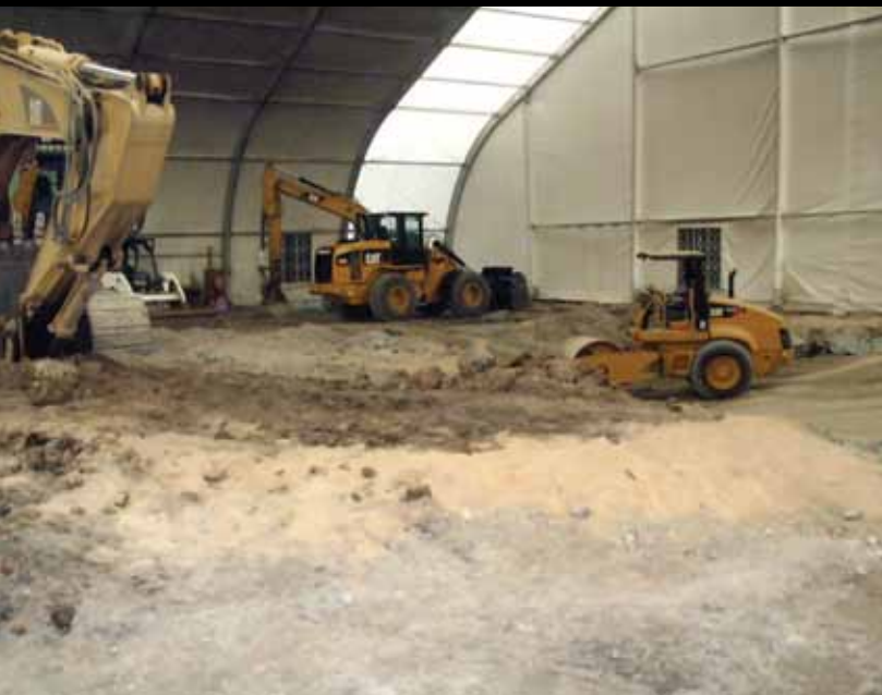
Project: Manufactured Gas Plant Site Remediation Location: Moberly, Mo. Client: Ameren Services
