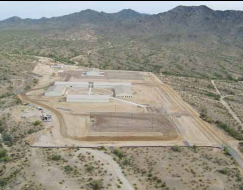
Project: Buckeye Readiness Center Location: Sonora Desert, Ariz. Client: Arizona Department of Emergency and Military Affairs
