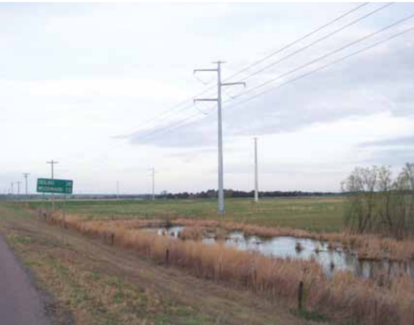
Project: WindSpeed Transmission Project Location: Oklahoma Client: OG&E
