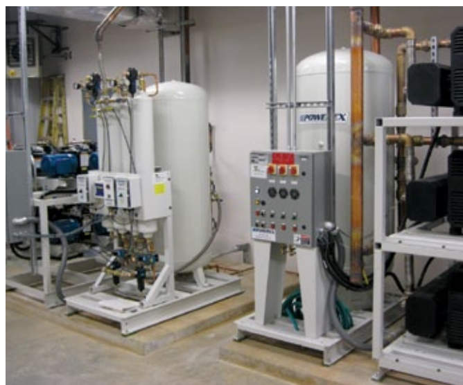
Medical gas equipment is part of the CUP project and includes medical air compressors and vacuum pumps that supply medical gases to the interim hospital.
