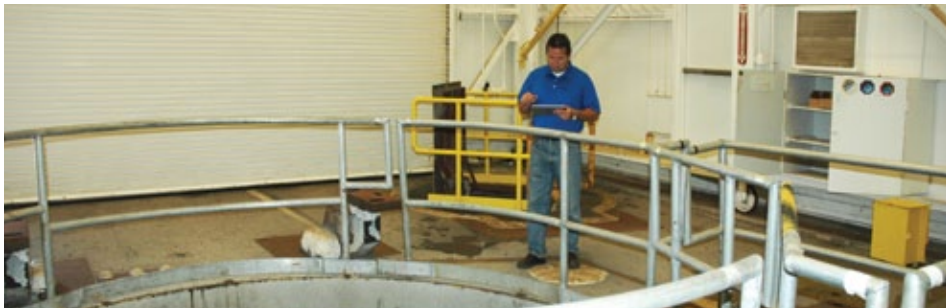
Perry Ryan, project manager, peers into a launch silo near Vandenberg Air Force Base in California. Plans call for all 103 launch tubes in the contract to absorb a combined total of 58,892 tons of fill — material weighing as much as a fleet of nearly 20,000 bulldozers.
